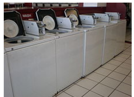
General Electric Filter-Flo top loading, vertical axis machines in laundromat. The pans on the inside of the lid are placed atop the agitator and wash water is pumped through the perforated pans to collect lint. (California)
