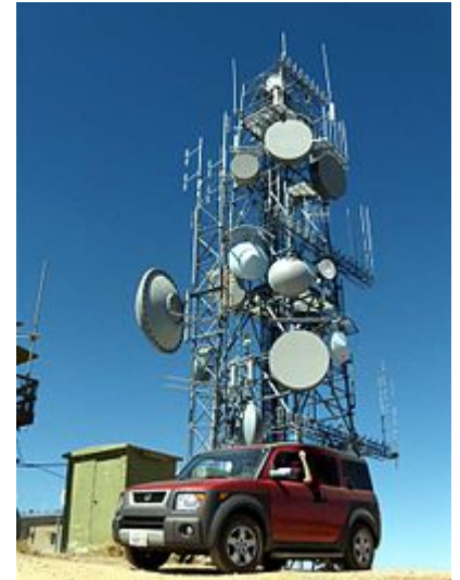
A telecommunications tower with a variety of dish antennas for microwave relaylinks on Frazier Peak, Ventura County, California.
