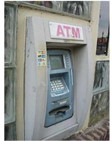
ATMs that are exposed to the outside must be vandal- and weather- resistant.
