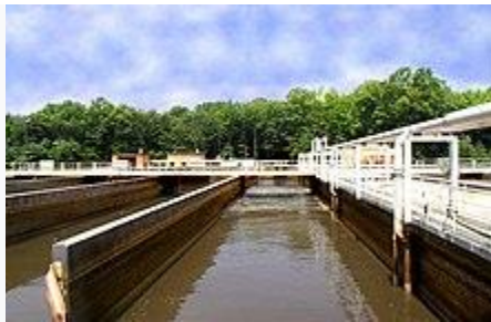
Nitrification process tank
