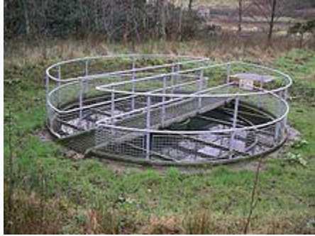
Secondary clarifier at a rural treatment plant
