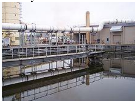
Primary treatment tanks in Oregon, USA
