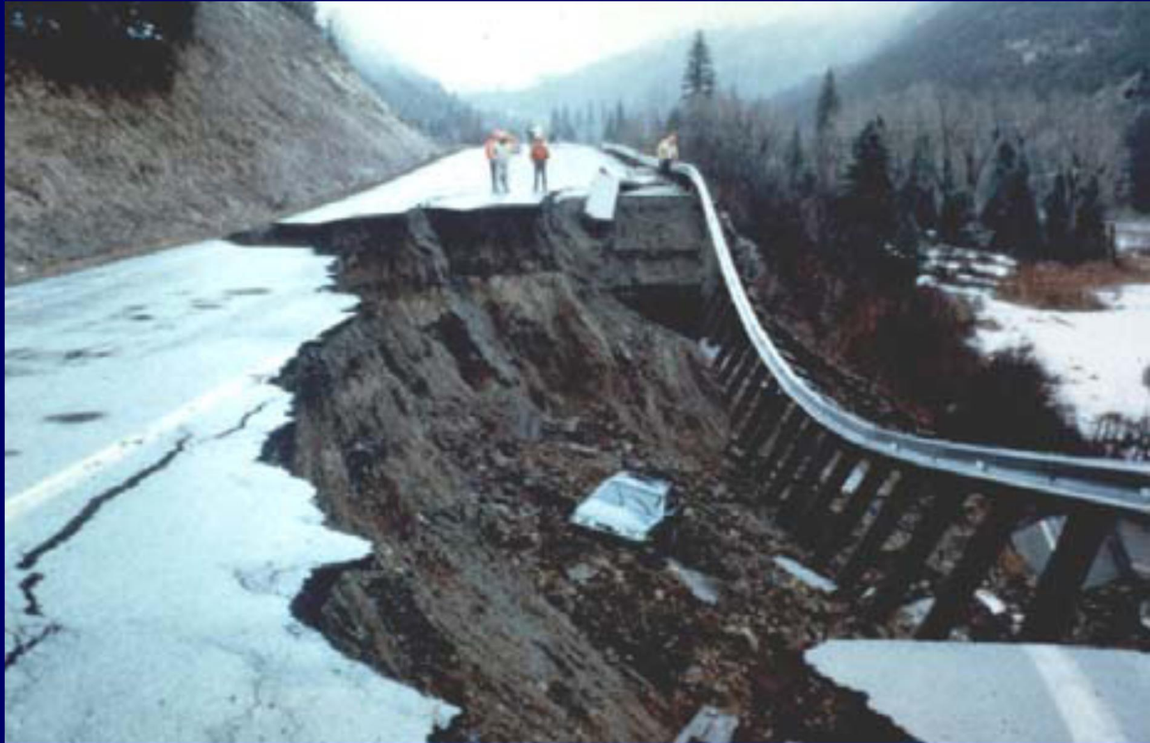
Slump in McClure Pass, CO.
