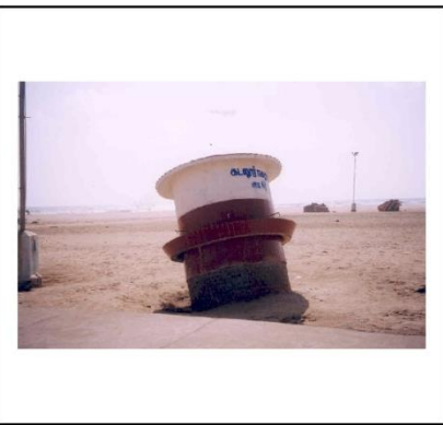
Collapsed drinking water tank - Cuddalore
