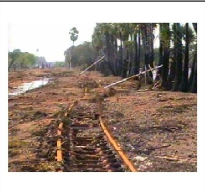
Washed away railway track - Nagore
