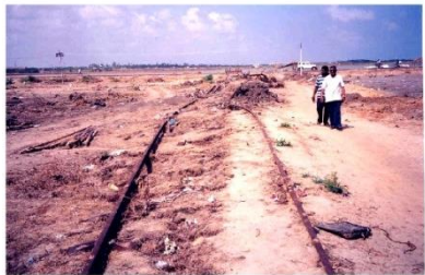
(E) Collapsed railway line - Nagore railway station
